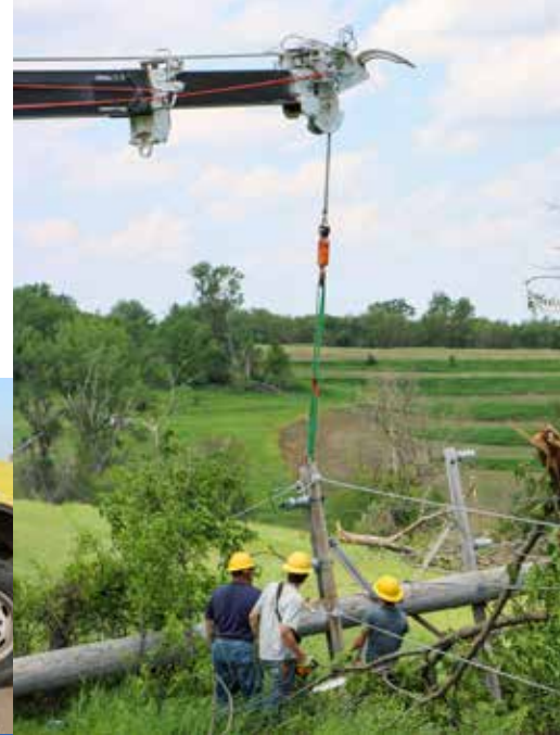
▶ Crews worked to lift a broken transmission pole in CIPCO's service territory.
